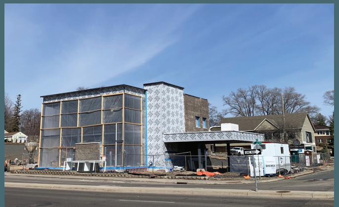
Bremer Bank under construction in St. Louis Park across from The Shoppes at Knollwood.
